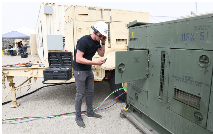
Figure 1-3. A User Wears an AR Headset to Speak to Someone in San Diego for Help With Fixing a Generator (Source: White [6]).
